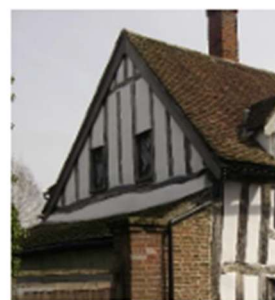
The images left show the north gable above the lean-to roof, the panels removed, and the finished work.
