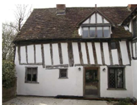
The images left show the rear elevation defective panels marked with red crosses, and the finished work.
