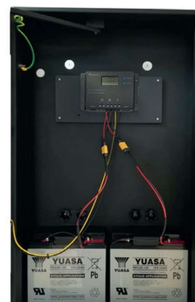
2 batteries and Solar Charge Controller
