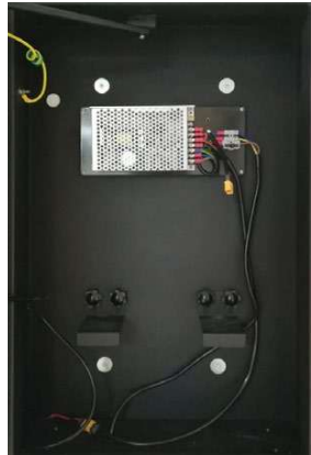
Optional batteries for intermittent power supply.
