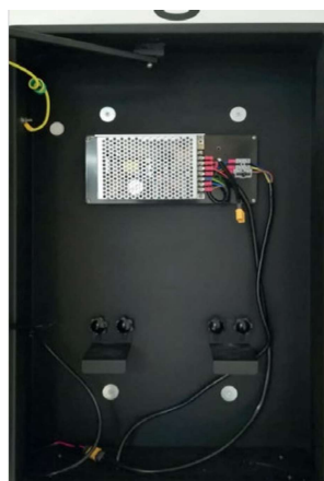
Optional batteries for intermittent power supply.
