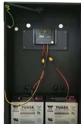
2 batteries and Solar Charger Controller
