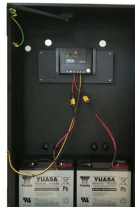
2 batteries and Solar Charger Controller
