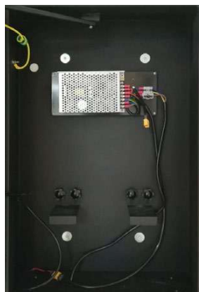
Optional batteries for intermittent power supply.
