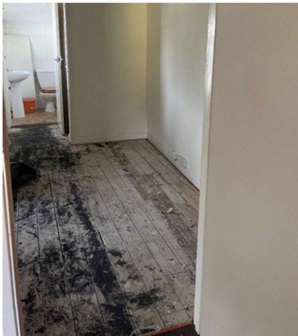
Photo Showing Modern Pine T&G Flooring From New Stair Void To Be Re-used To Infill Existing Stair Void
